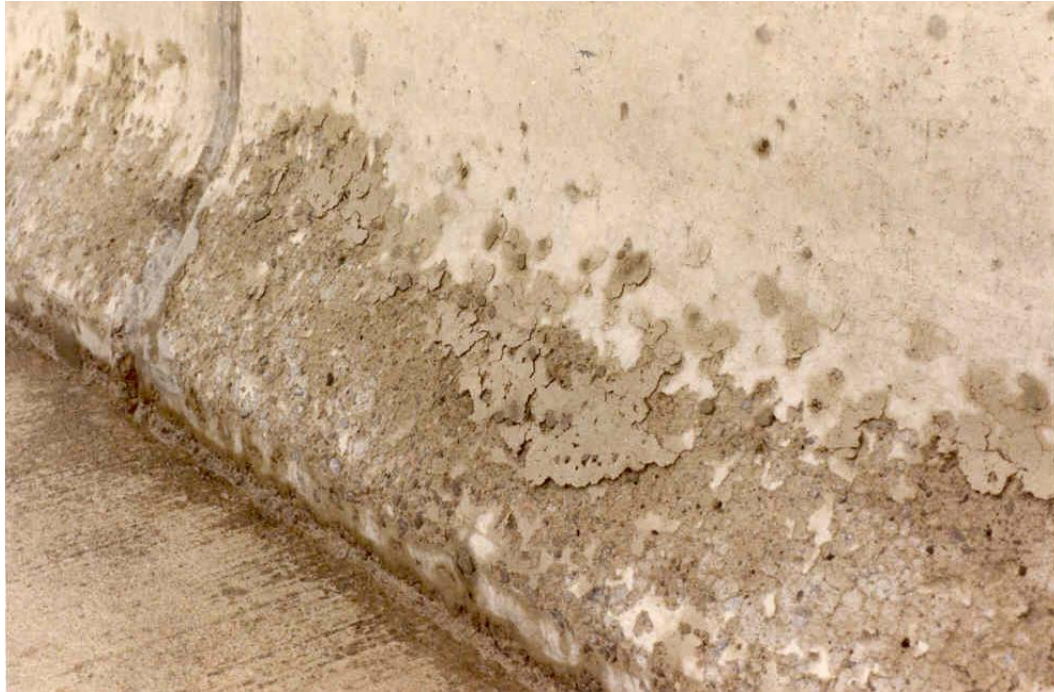
FIGURE 5 Example of Severe Scaling
